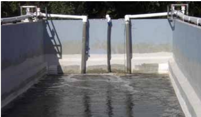
Fig. 13. Wastewater treatment system at Catapereiro
